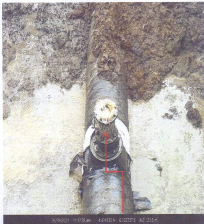
FIG.2 Incident facility after exposure 6" inch valve
